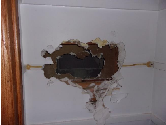
Figure 69: Wall damage (likely selective demolition) at first floor. Sept. 2021.
