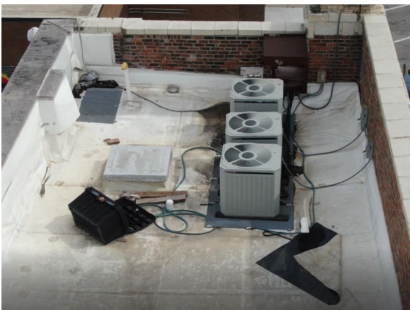
Figure 44: Mechanical units on roof, view south. Sept. 2021.
