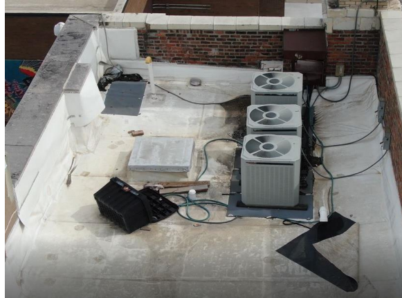
Figure 100: Rooftop units. Sept. 2021.
