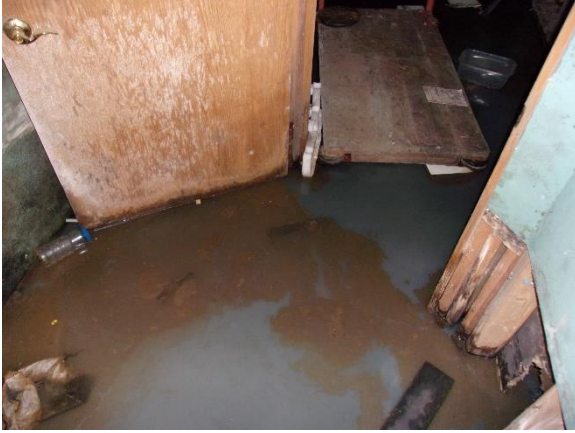
Figure 73: Typical conditions at basement. Sept. 2021.
