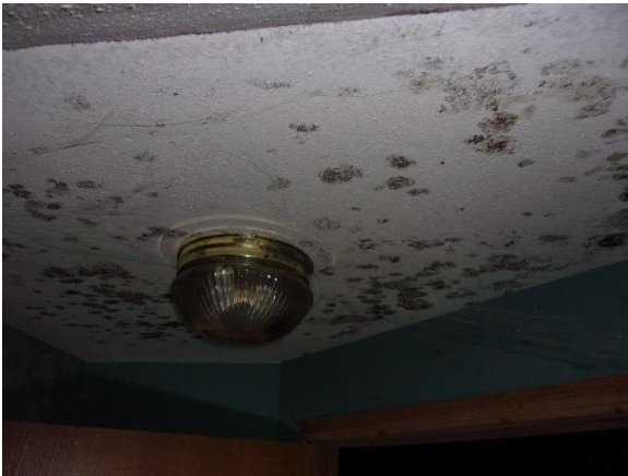
Figure 80: Typical ceiling conditions at basement. Sept. 2021.
