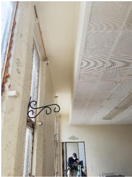
Figure 84: Second floor dropped ceiling set back to maintain original window openings. Sept. 2021.
