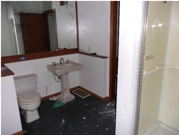
Figure 111: Non-accessible plumbing fixtures. Sept. 2021.
