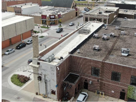
Figure 19: Roof and Related Features: Roof is low-sloped, not visible from pedestrian right-of-way. View southeast. Sept. 2021.
