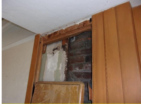
Figure 70: Structural brick wall exposed behind finished walls at first floor at east wall. Sept. 2021.
