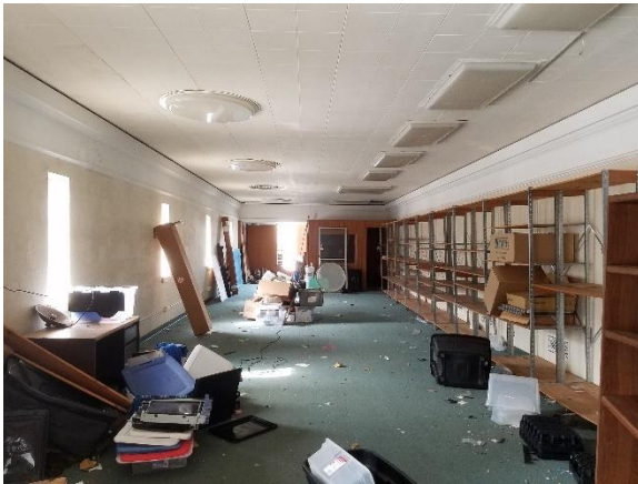
Figure 106: Lighting at first floor. Sept. 2021.
