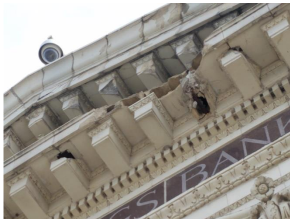
Figure 23: Materials: Extensive terra cotta details and cladding are a prominent feature. Limestone, granite and glazed brick make up the remainder of the exterior walls. View northwest. Sept. 2021.
