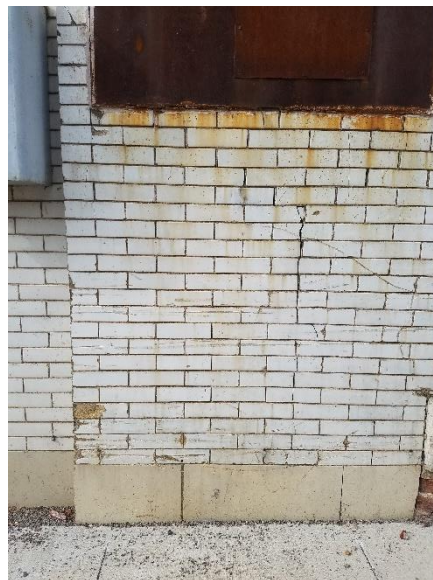
Figure 53: Typical conditions of glazed brick at alley elevation. North elevation. Sept 2021.
