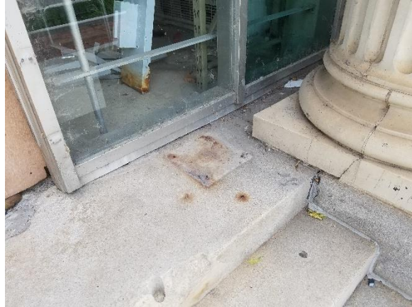
Figure 58: Storefront condition and main entrance. View northeast. Sept. 2021.
