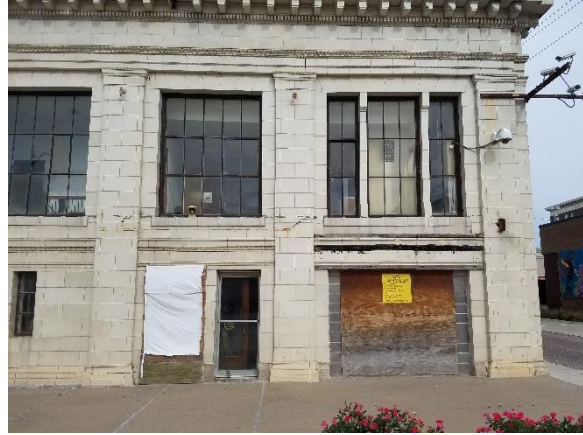
Figure 110: Small step at north end of east elevation. Sept. 2021.
