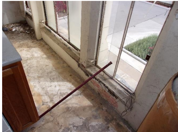
Figure 78: Exposed sub-flooring at second floor. Sept. 2021.
