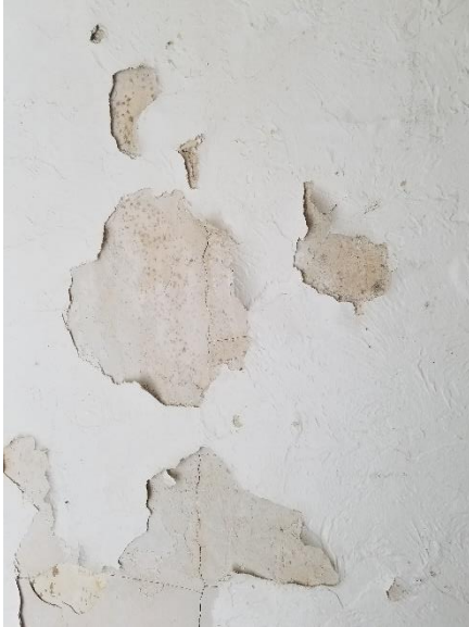
Figure 87: Peeling paint conditions at first floor. Sept. 2021.
