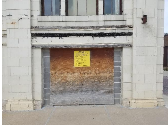
Figure 55: Typical condition of foundation wall at openings, gray limestone. Sept 2021.
