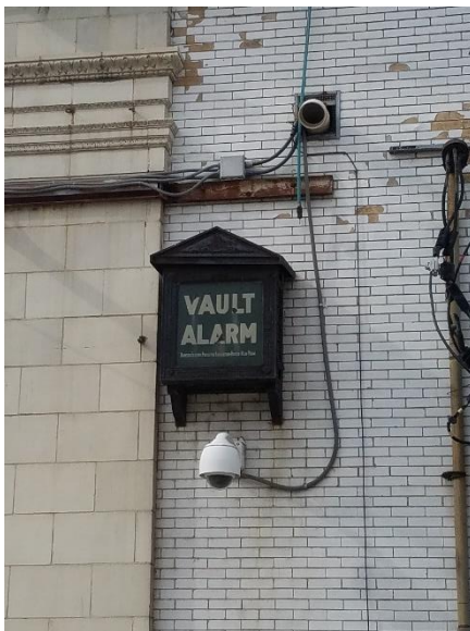
Figure 52: Vault alarm located on alley elevation. North elevation. Sept 2021.
