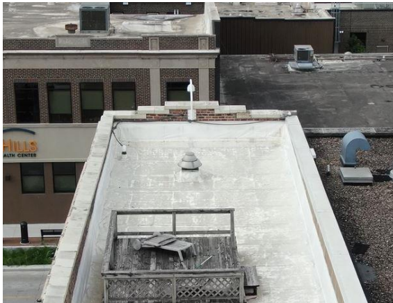
Figure 99: Rooftop vents. Sept. 2021.
