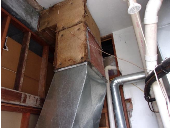
Figure 98: Mechanical ducts, second floor. Sept. 2021.
